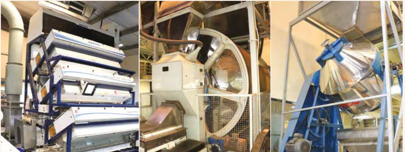
Tea mixing & refining plant
